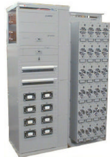
Power Distribution Frame and 1200a Charger Bay
